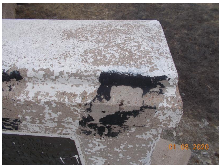
Paint sample M-21-C-LP02. The black paint on the concrete and metal girders is considered lead-based paint.
