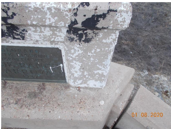
Paint sample M-21-C-LP01. The white paint on concrete is considered lead-containing paint.
